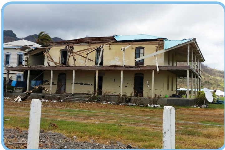
Damaged Classroom – St. Johns College in Levuka
